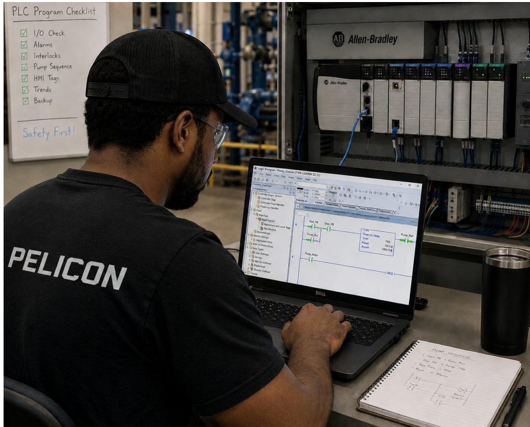
Illustrative image: PLC programming and commissioning
