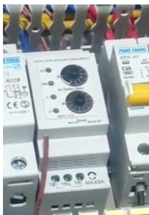
Three-phase controller in a control panel
